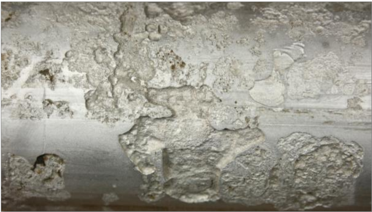
Oxygen pitting after cleaning
