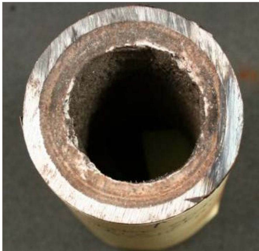
1.5" diameter wall tube from watertube boiler. Layered phosphate and iron deposits from years of multiple feedwater hardness and internal water treatment chemistry upsets.
