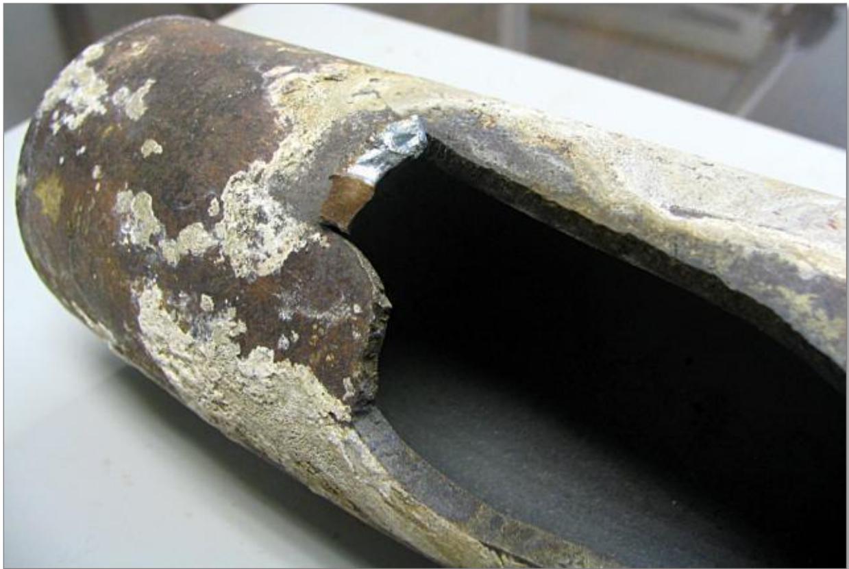
Hydrogen damage to high pressure boiler tube
