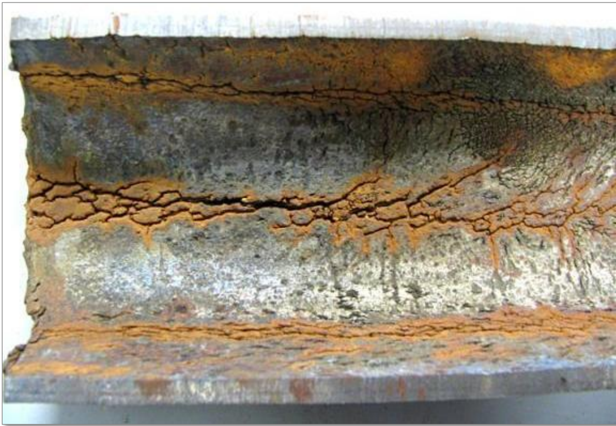
Internal tube surface cracks developed under coincident external surface weld overlay to repair a tube leak.
