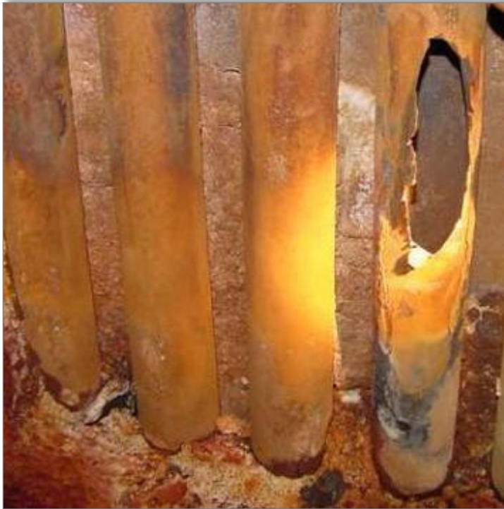
Flame impingement – rear wall
