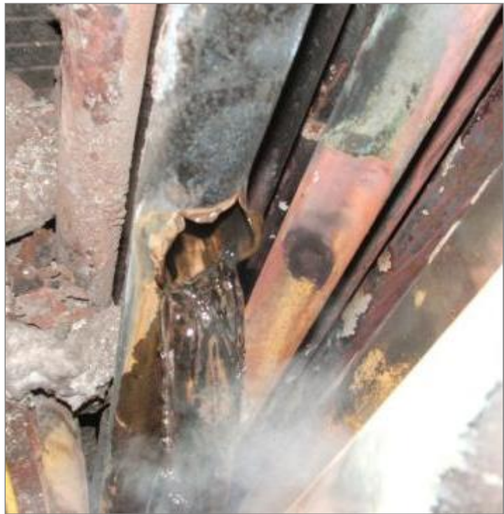
Flame impingement – back corner of furnace
