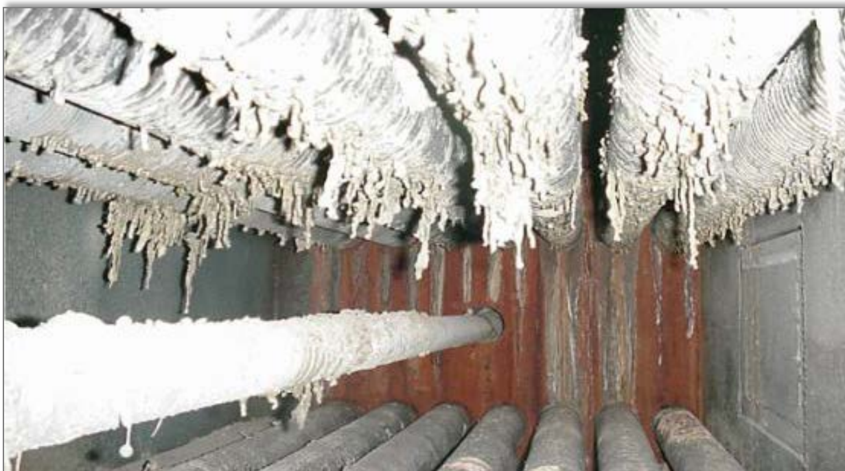
Section of fouled, finned economizer tubes
