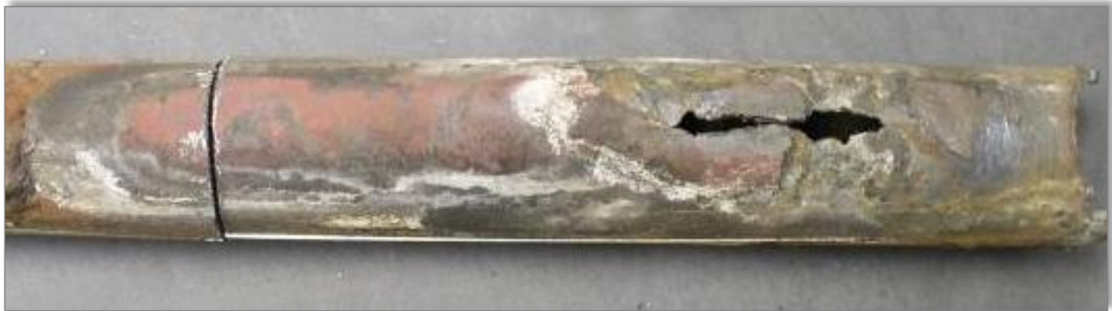
Tube surface damage resulting from flame impingement
