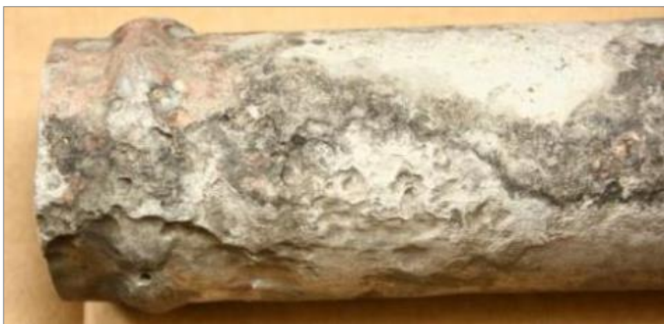
Close-up after cleaning, showing external surface metal loss
