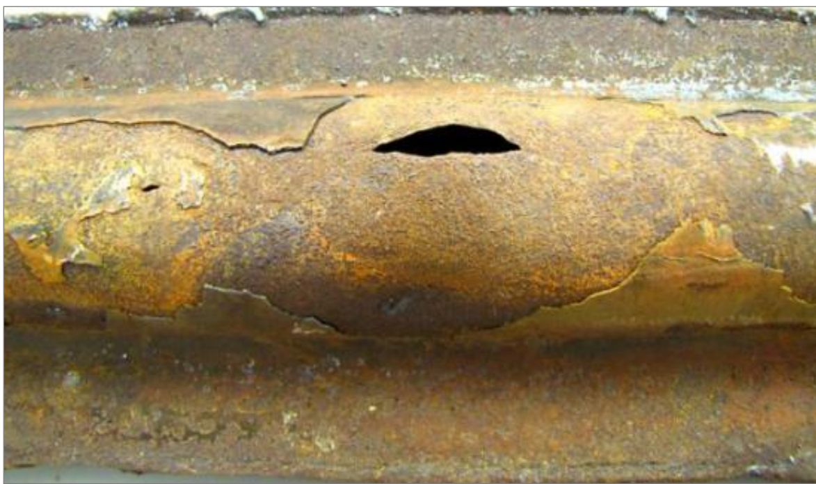
Tube metal creep and failure due to overheating from flame impingement
