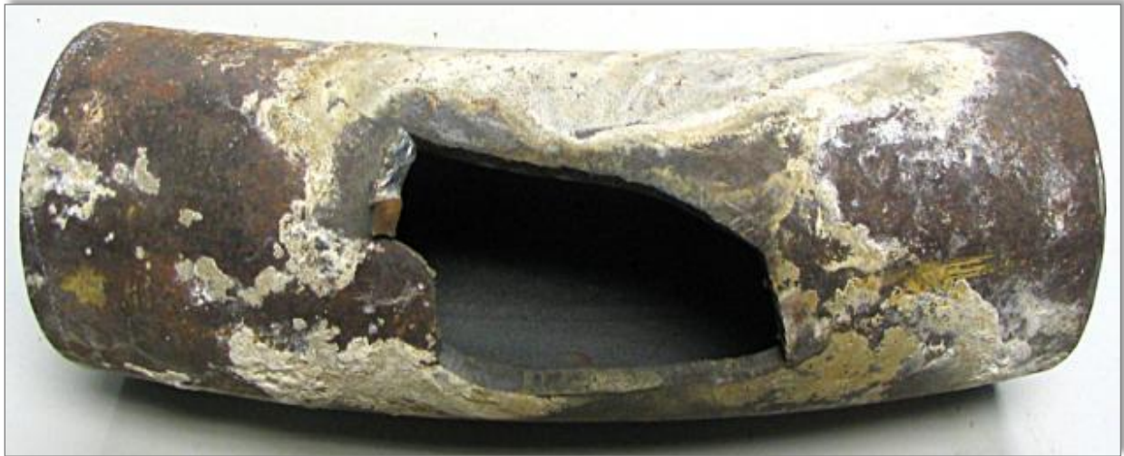
Hydrogen damage to high pressure boiler tube
