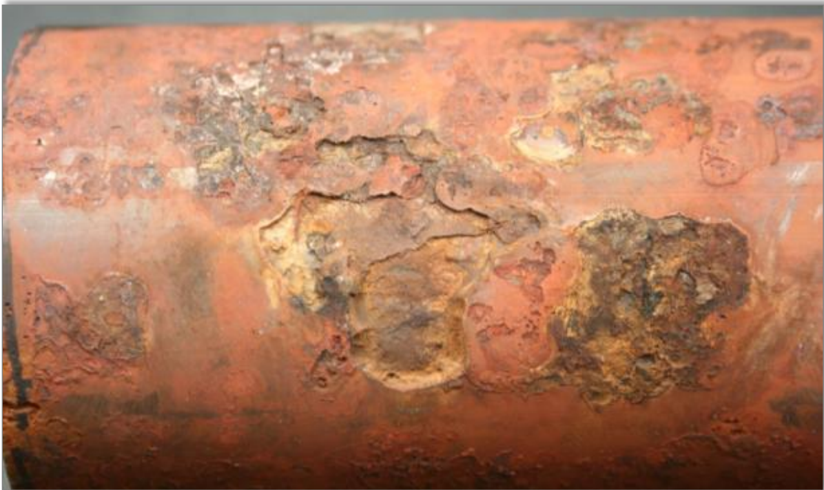
Oxygen pitting before cleaning – resulting from oxygen intrusion during offline storage
