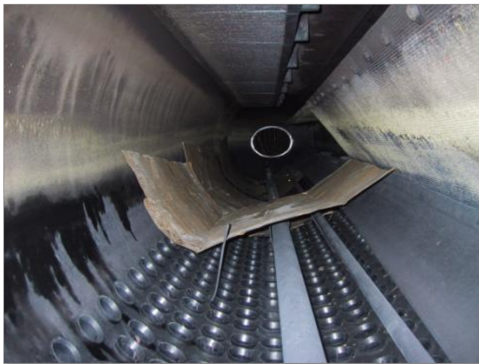
Clean steam drum downcomer tubes, deposit fouled steam diffuser screen and boiler drum sidewalls
