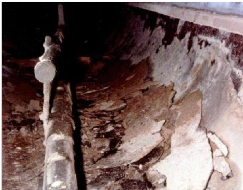
Steam drum: Extreme, excessive quantity of scale and surface deposits
