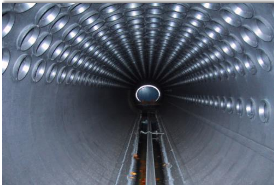
Clean mud drum and tubes
