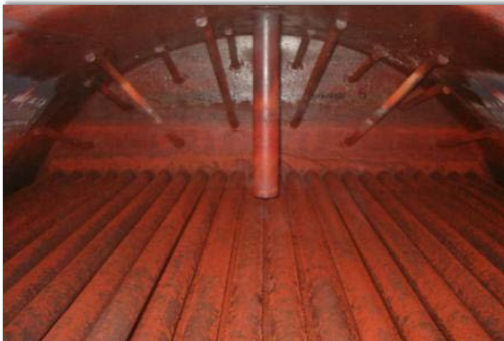
Tubes showing surface iron deposits and flash rusting
