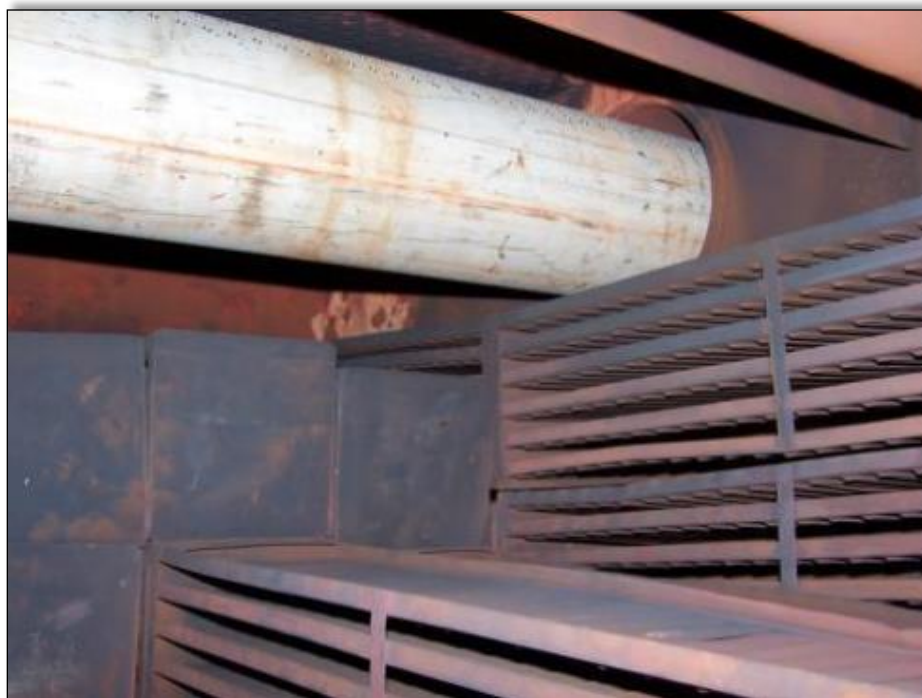
Distorted and collapsed deaerator trays
