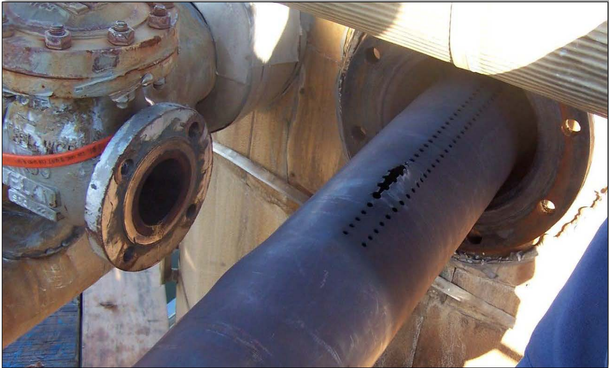
Deaerator inlet header spray pipe failure
