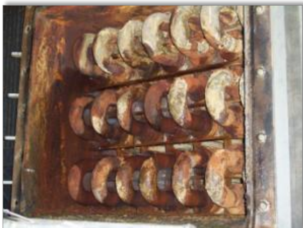
Return bends outside the flue gas envelope.
