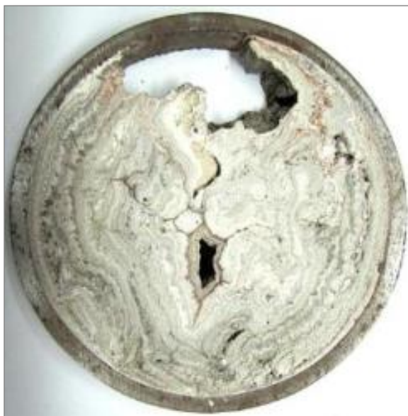
Deposits in 6 inch diameter steam line due to long term intermittent boiler water carryover
