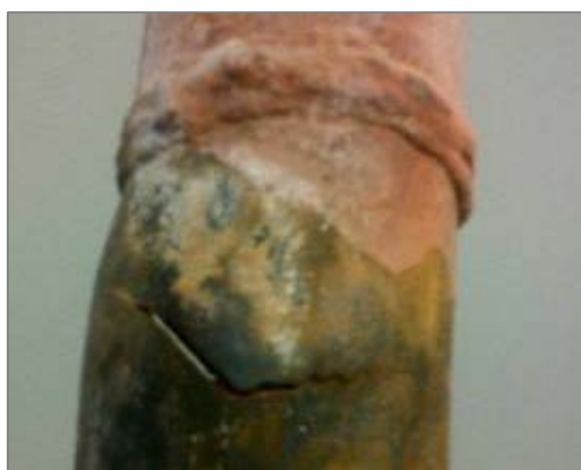
Additional surface crack formation
