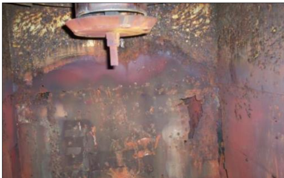
Deaerator spray zone corrosion on SS shell due to high chlorides
