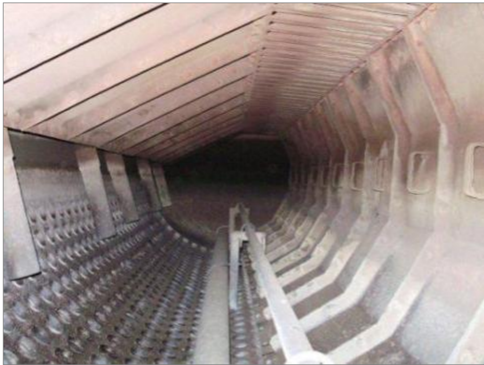
Steam drum surface after two years on an internal cleanup program
