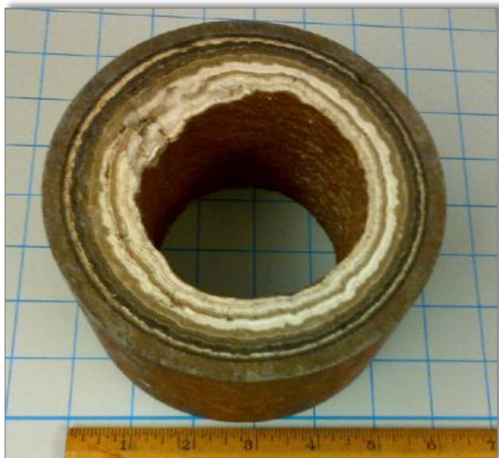
Feedwater line deposits – multiple hardness upsets in 100 year old system
