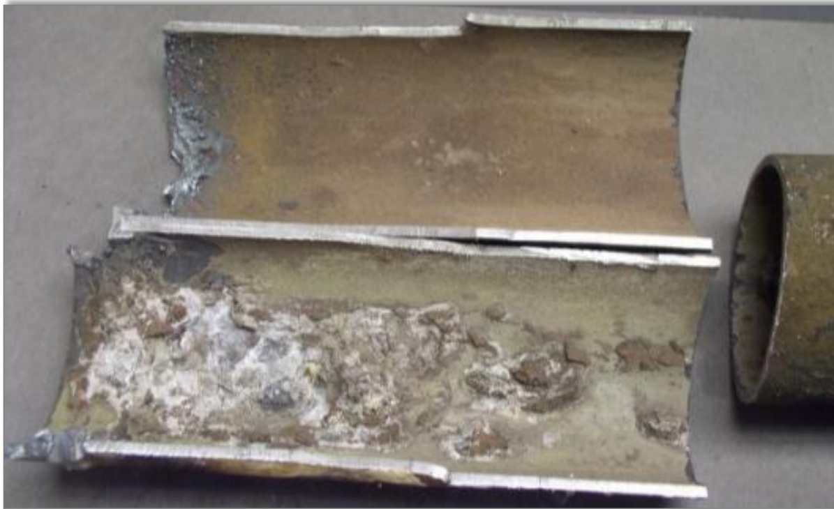
Inclined overhead boiler tube – deposits on the inside (bottom) surface facing the furnace
