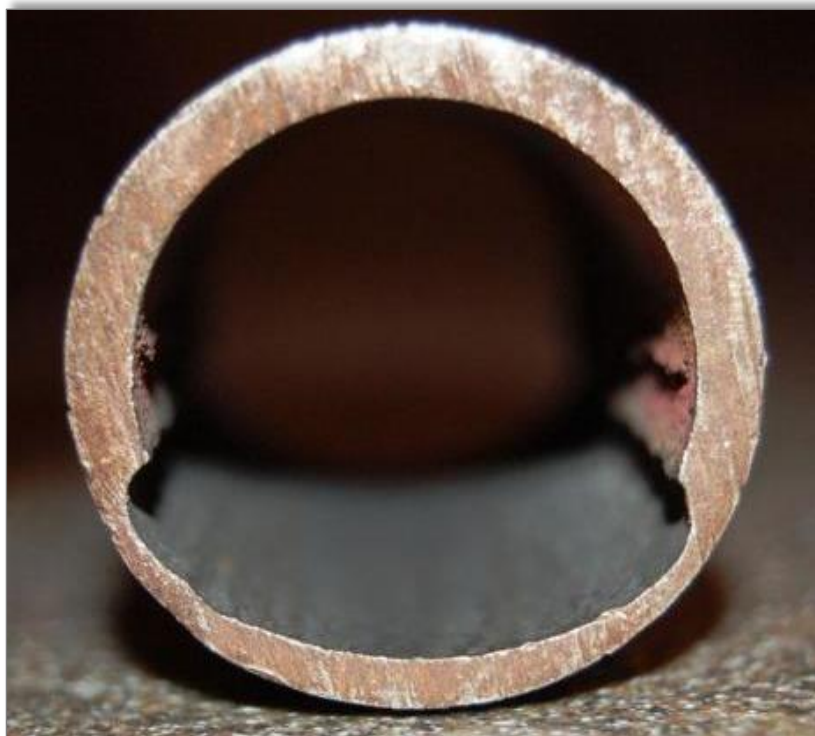
Corrosion due to low pH (from carbonic acid) at the bottom of a condensate return line
